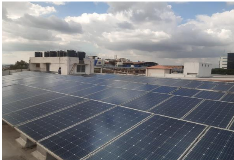
Figure 3-1: Solar rooftop PV system
