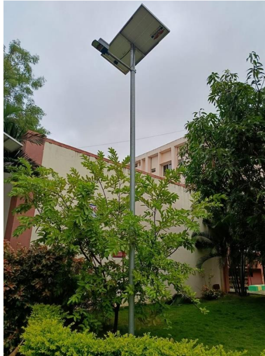
Figure 3-7: Solar LED Street lights
