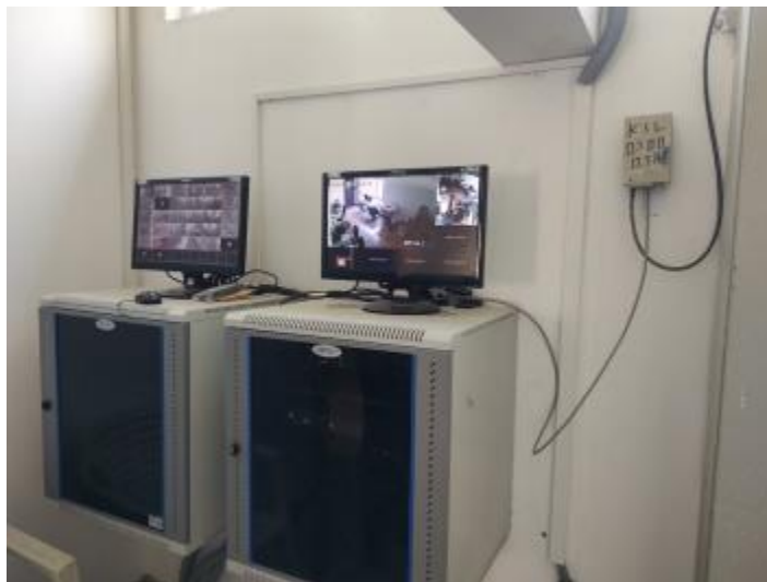
Figure 3-13: Use of LED monitors in server room
