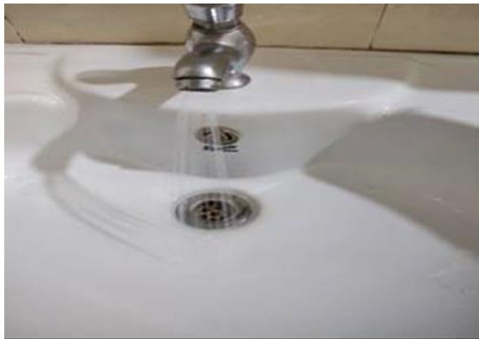
Figure 3-16: Low flow taps installed in the college
