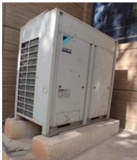
Figure 3-11: Energy Efficient Air Conditioner
