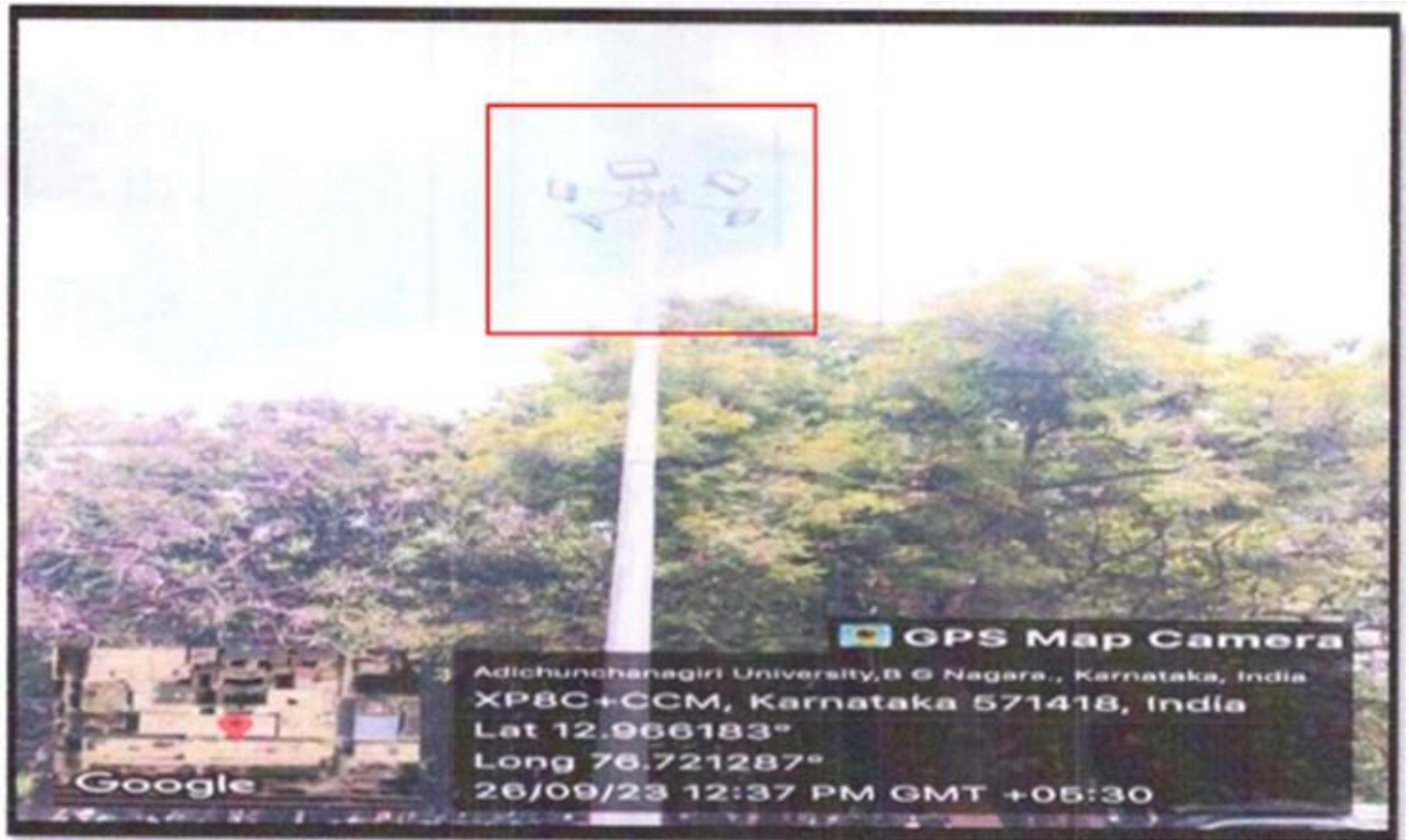
Figure 3-8: LED Street light Fixture
