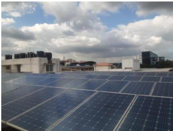
Figure 3-5: Sample photo – SRTPV system
