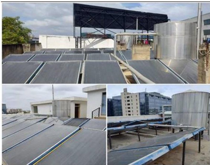
Figure 3-9: Use of Solar Water Heater
