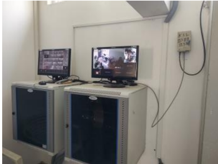
Figure 3-13: Use of LED monitors in server room
