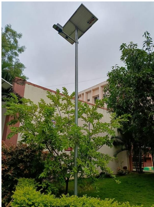
Figure 3-7: Solar LED Street lights
