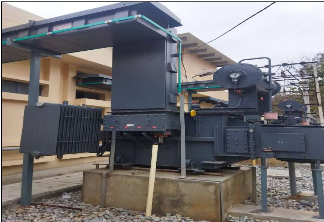
Figure: - 1000 KVA Transformer Photographs
