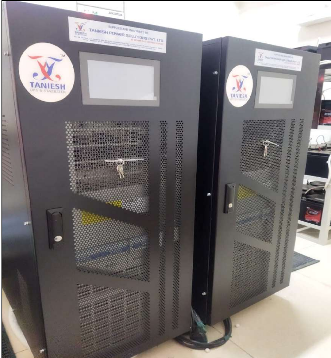
Figure: - UPS System for Emergency Power failure
