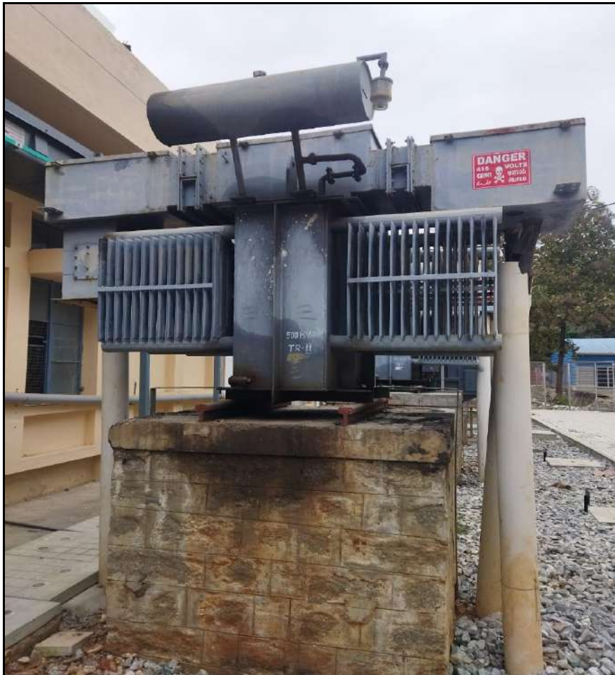
Figure: - 250 KVA Transformer photographs
