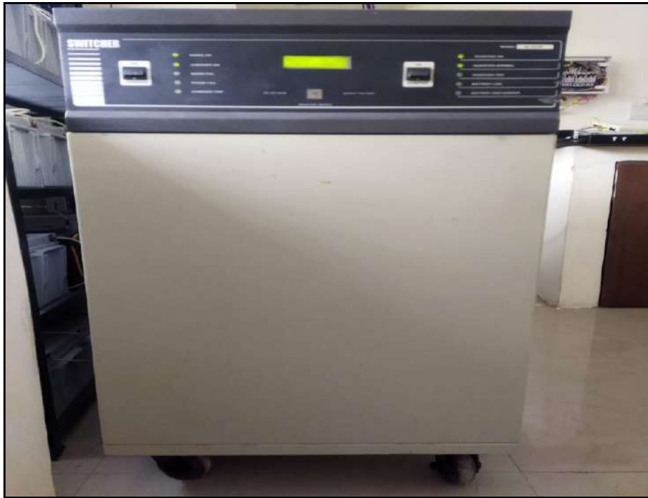
Figure: - UPS System for Emergency Power failure
