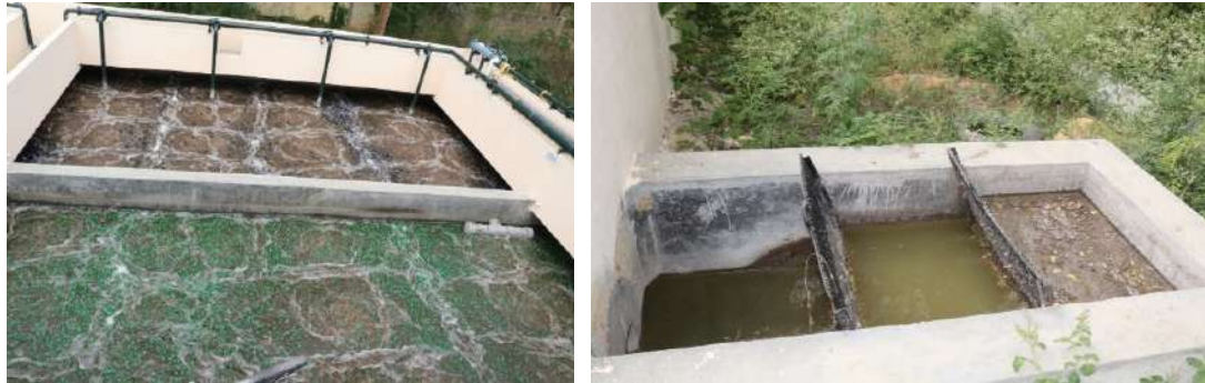
MBBR unit in Sewage Treatment Plant. Screening unit in Sewage Treatment Plant.
